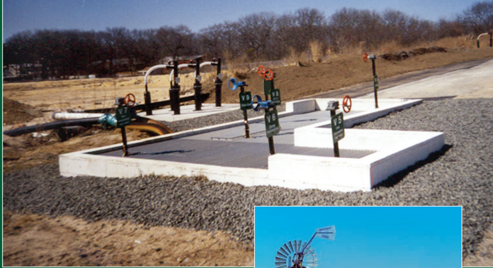
Town of Islip Resource Recovery Agency, Blydenburgh Landfill Gas System Manifold Valve Pit.
